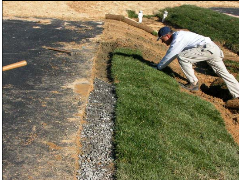
Figure 5.6 A gravel verge precedes a sod filter strip leading into this bioretention area (rain garden).
