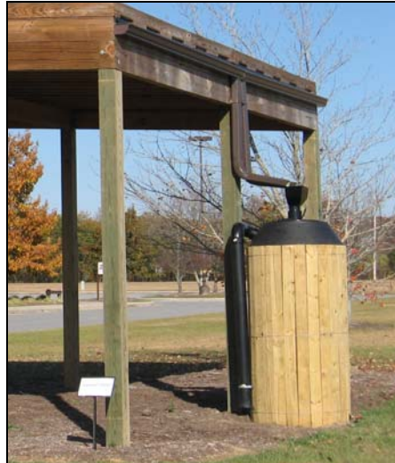
Figure 7.3 300-gallon cistern in Greenville, N.C.
