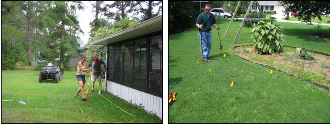
Figures 6.5a and 6.5b Mark wetland area prior to excavating the area
