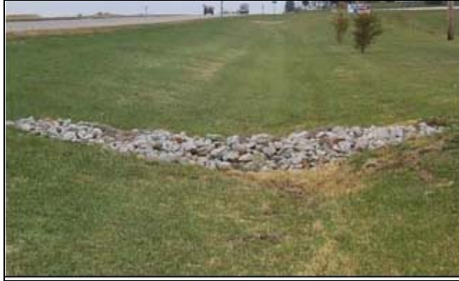
Figure 6.4 Swale with check dam constructed of stone (Source – USDA – Natural Resource Conservation Service – Illinois)
