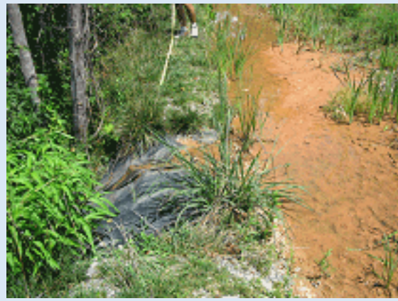
Figure 3. Failure at level spreader constructed with ABC stone
