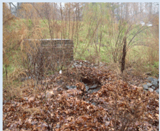
Figure 7: Sediment and debris build-up after approximately 4.5 years of operation
