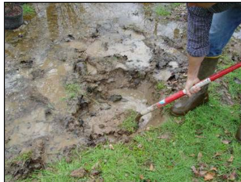
Figure 3.10 Obvious wet conditions in this location lead to selecting a backyard wetland as a stormwater BMP
