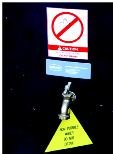
Figure 7.3 Warning signs on a cistern to prevent human intake of the stormwater
