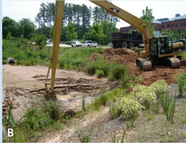
Figure 2. Inspection (A) of sediment depth and cleaning or "dipping" (B) of forebays. A long boom on the excavator is sometimes essential to access sediment collected in the middle of the forebay.
