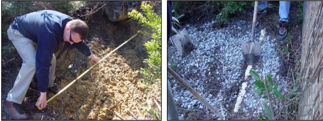
Figures 7.8a Cistern site preparation and b. Preparing the gravel support base.
