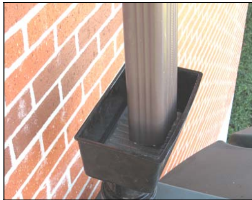
Figure 7.5 Debris filter just below gutter downspout
