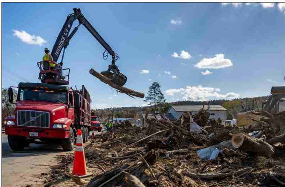
Crews collecting storm debris after Helene. Contributed by Buncombe County.
