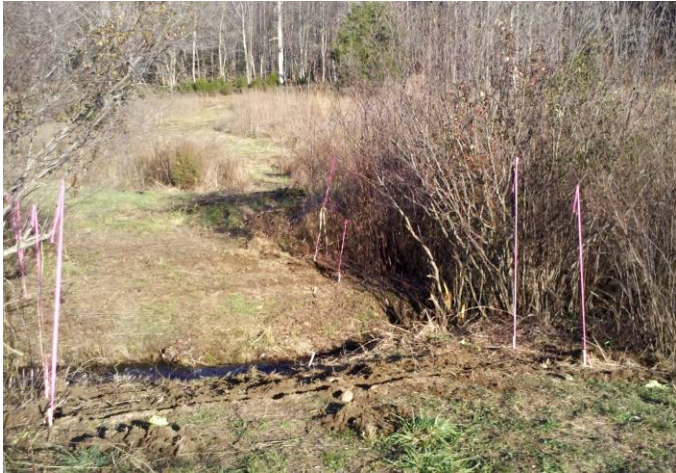
Crossing location prior to bridgemat installation. Vegetation disturbance was kept to a minimum. Soil erosion was mitigated by installation of silt fence.
