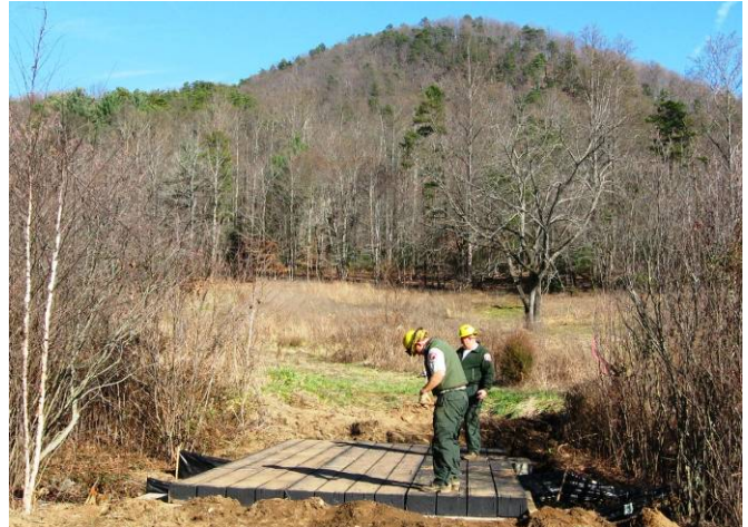
Bridgemat crossing installed. The State Forest property on the opposite side of the stream crossing is now accessible.
