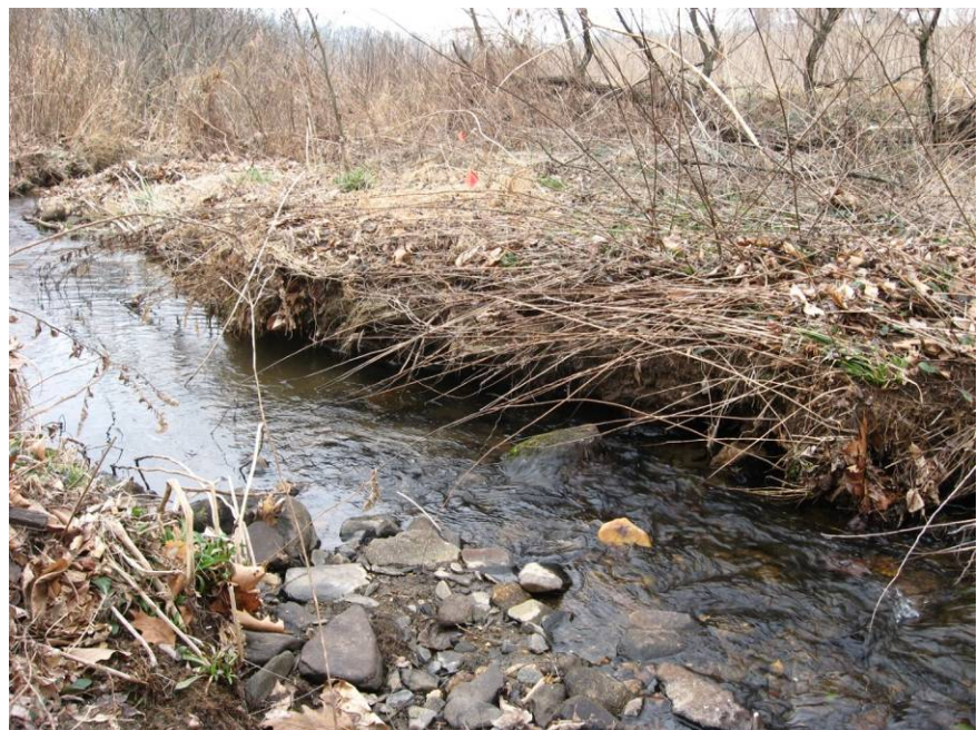
Photo at right: February 22, 2011. This short segment of right bank has been partially undercut.
