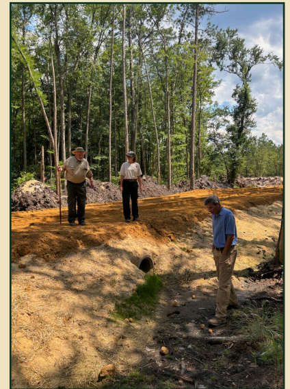
NCFS and U.S. Army Corps of Engineer representatives on a forest road during the construction phase.
