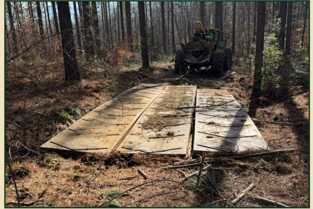
A set of temporary bridges placed at a ditch crossing on a thinning operation.
